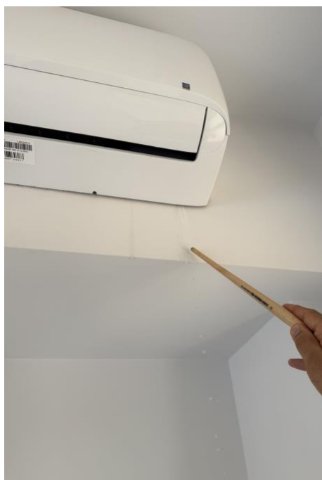
Figure 34. Water leakage visible below a ground-floor split air-conditioning indoor unit.
