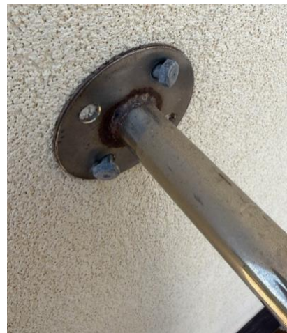
Figure 12. Roof-access ladder fixing plate with incomplete bolting.
