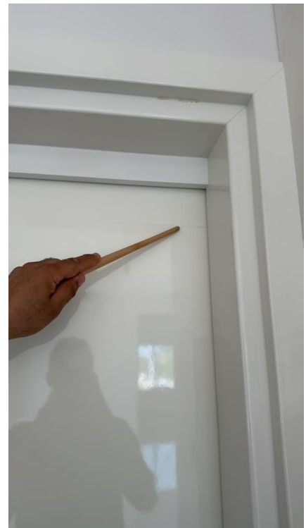
Figure 27. Contact marking at the upper sliding-door interface.
