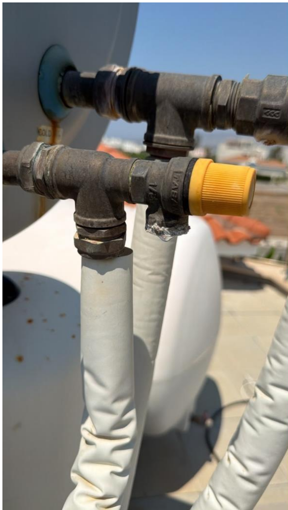
Figure 60. Visible droplet at the solar hot-water valve fitting.
