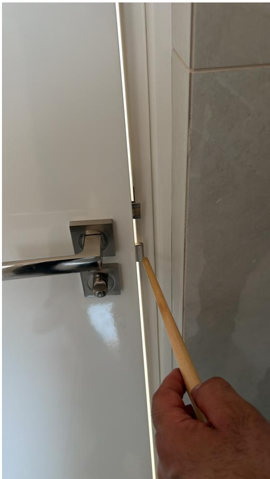
Figure 37. Guest WC door hardware requiring adjustment and completion.
