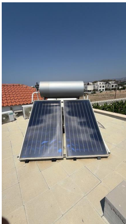
Figure 63. Roof-mounted solar hot-water collectors and storage tank.
