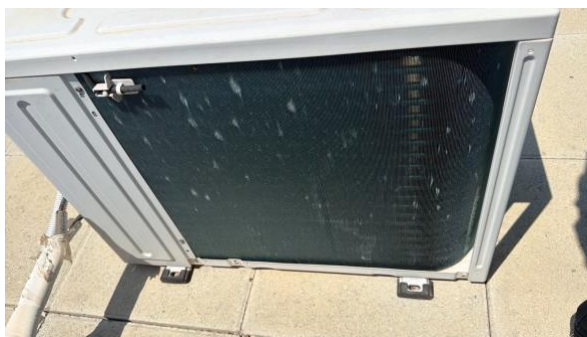
Figure 56. Localized damage to condenser coil fins.
