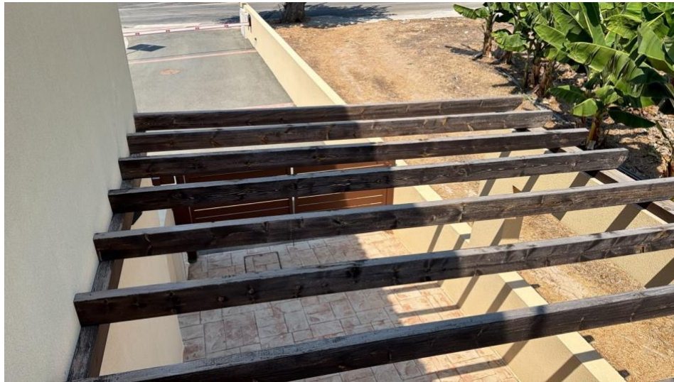
Figure 7. Weathered timber pergola requiring renewed protective finish.
