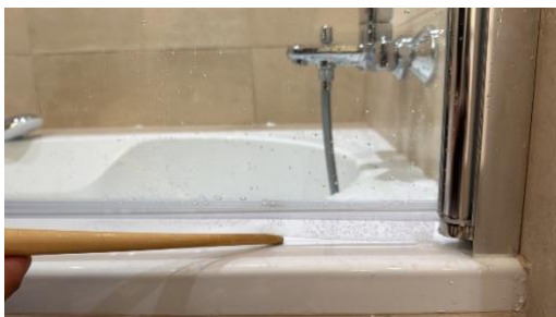
Figure 40. Water at shared-bathroom screen junction.
