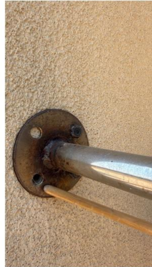
Figure 10. Close-up of a ladder wall fixing showing incomplete bolting arrangement.
