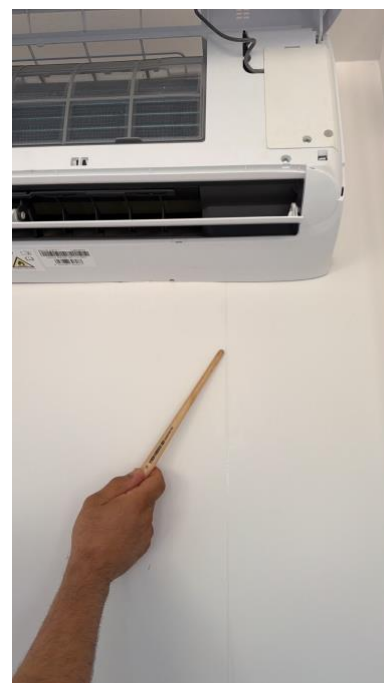
Figure 36. Additional ground-floor split air-conditioning unit inspected for condensate-drainage leakage.
