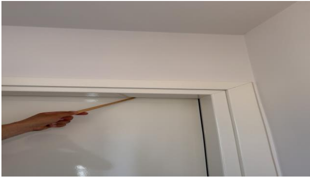
Figure 54. Third-bedroom door contacting the upper frame during closing.
