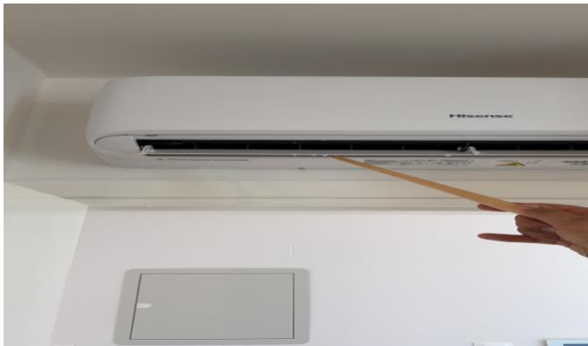
Figure 50. Middle-bedroom air-conditioning unit associated with the condensate drainage defect.
