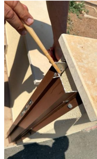
Figure 16. Open gap at the vehicle gate and boundary finishing junction.
