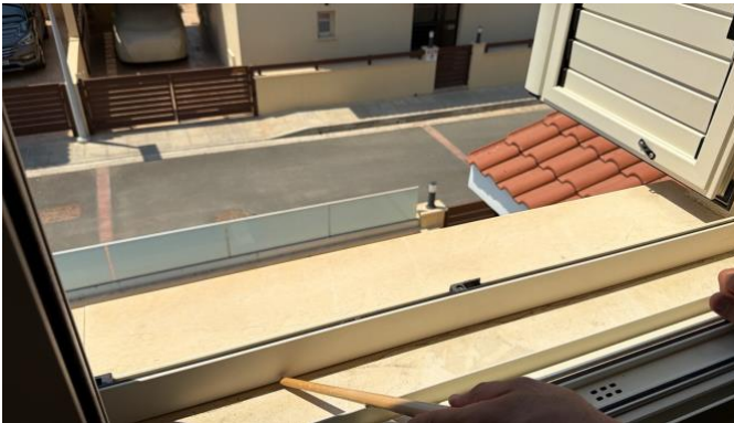
Figure 46. Middle-bedroom shutter frame with incomplete sealing at the lower junction.
