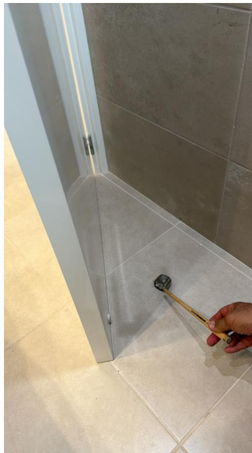
Figure 45. Floor-mounted door stop adjacent to the master-bathroom door.
