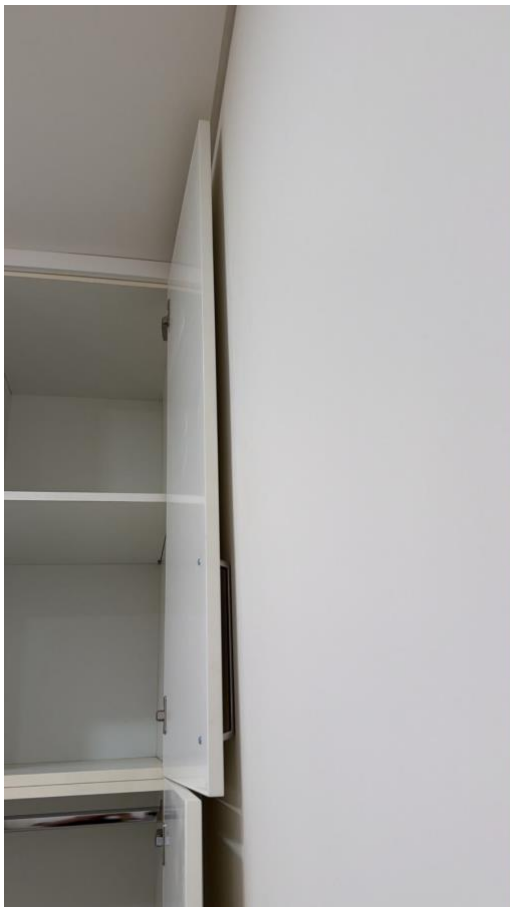
Figure 52. Wardrobe door with insufficient clearance to the adjacent wall.
