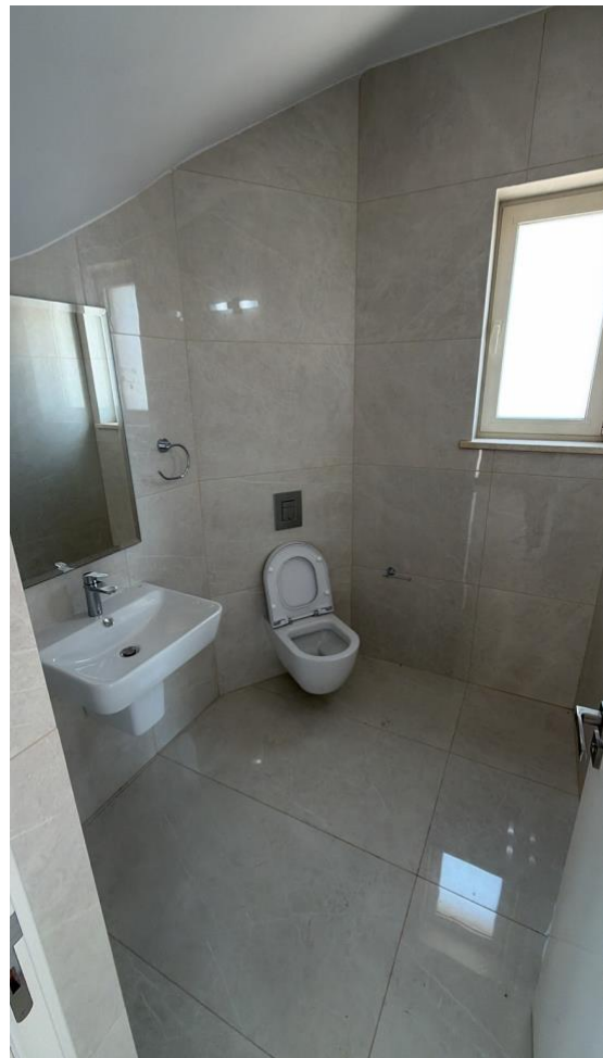
Figure 38. Overall view of the ground-floor guest WC and affected internal door.
