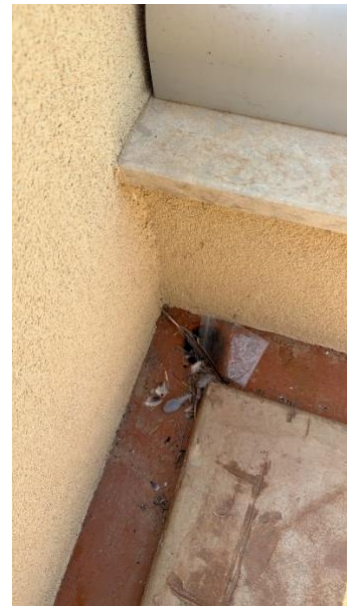
Figure 20. Further uncovered pool-area drainage opening with debris accumulation.
