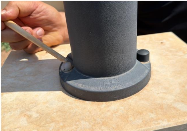
Figure 13. Missing protective screw cap at an external light fitting.
