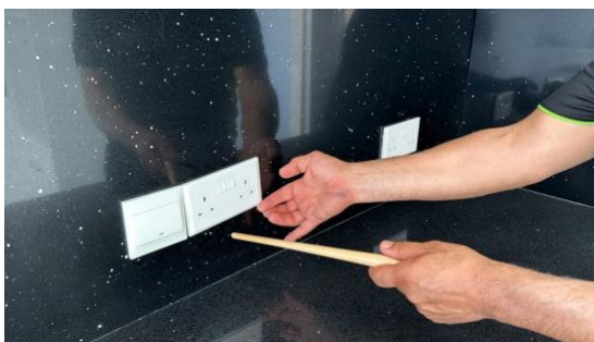
Figure 32. Loose kitchen electrical socket showing movement from the wall finish.
