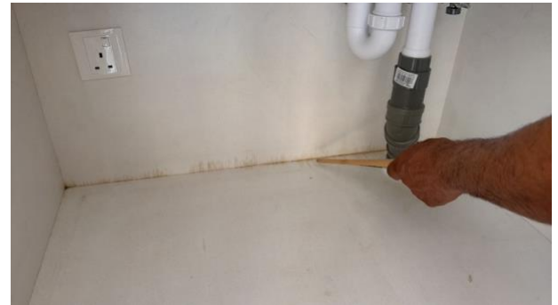
Figure 31. Yellow staining at the under-sink cabinet junction.
