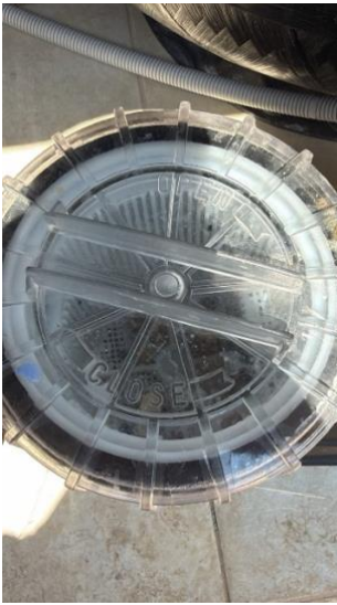
Figure 17. Debris visible within the pool filter basket.
