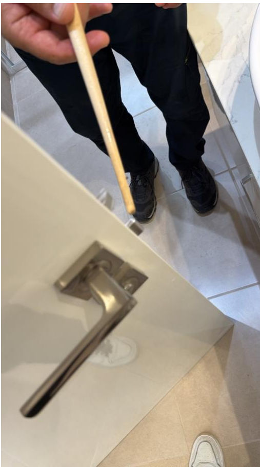
Figure 44. Master-bathroom door/lock requiring adjustment.
