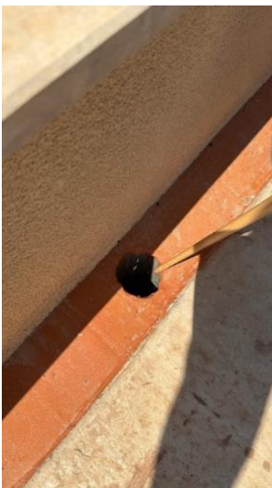
Figure 19. Uncovered drainage opening within the pool area.
