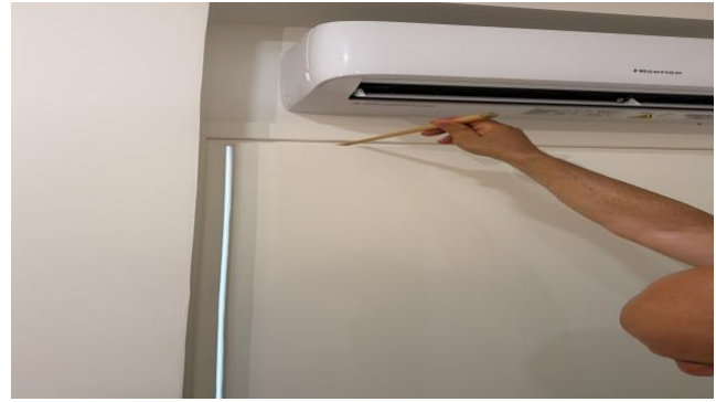
Figure 55. Further view of the third-bedroom door/frame interference.
