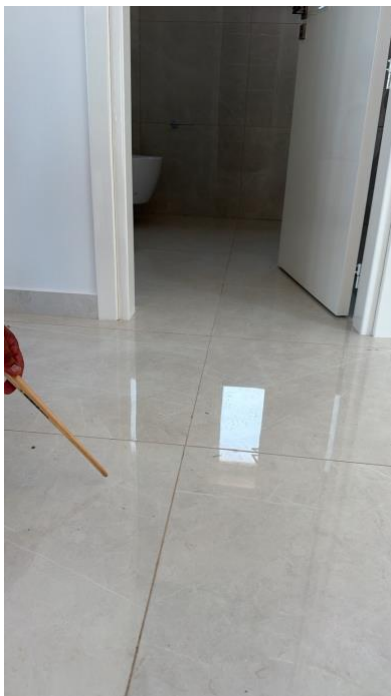
Figure 22. Tap testing of ground-floor tiles where hollow response was identified.
