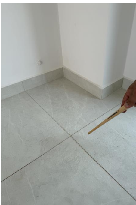
Figure 35. Residual water on the ground-floor finish associated with condensate leakage.
