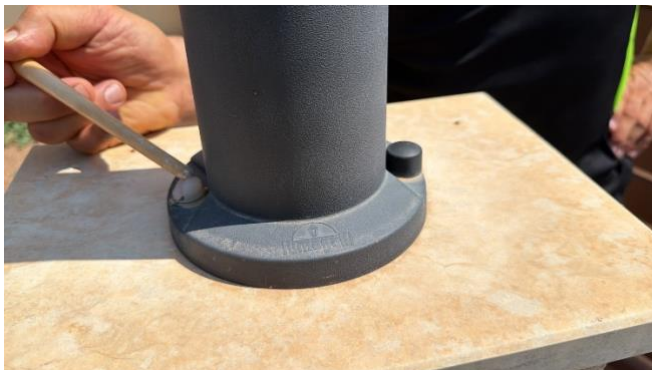
Figure 15. Further view of the missing protective screw cap at an external light fitting.
