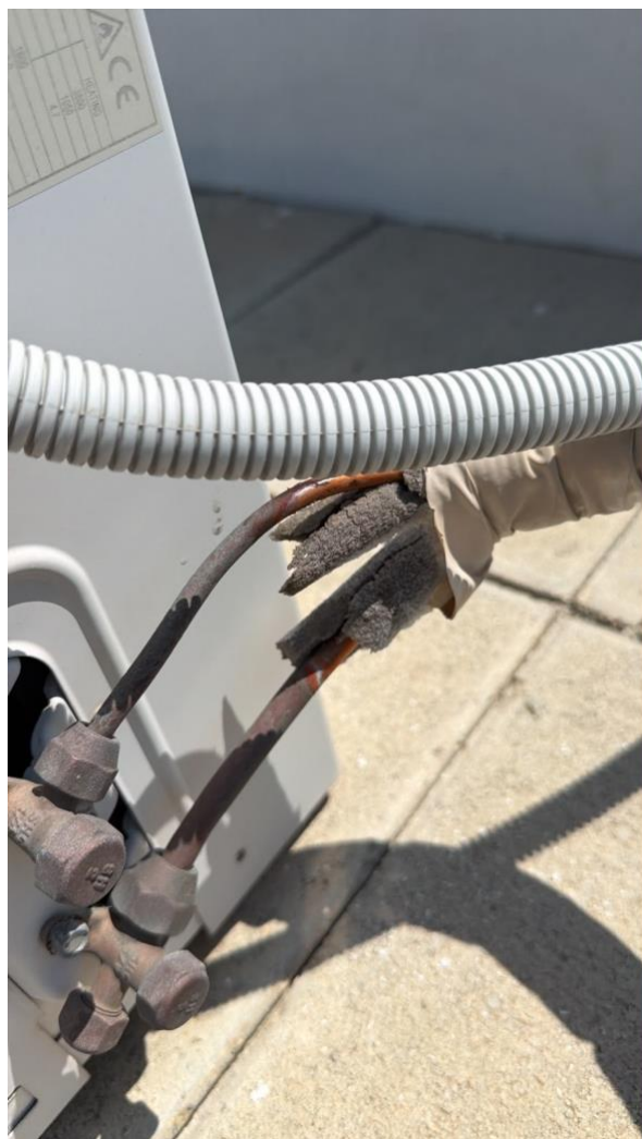
Figure 58. Deteriorated refrigerant-line insulation.
