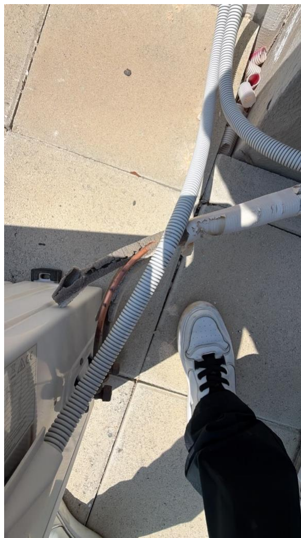
Figure 59. Exposed copper where insulation has deteriorated.
