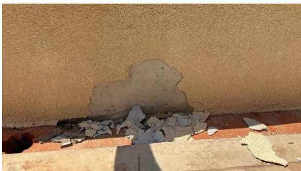
Figure 5. Localized delamination of textured exterior render.
