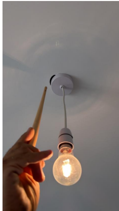
Figure 49. Gap around the first-floor ceiling light fitting.
