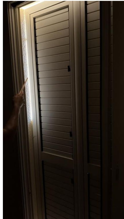
Figure 47. Visible daylight through an open side junction at the shutter-frame perimeter.
