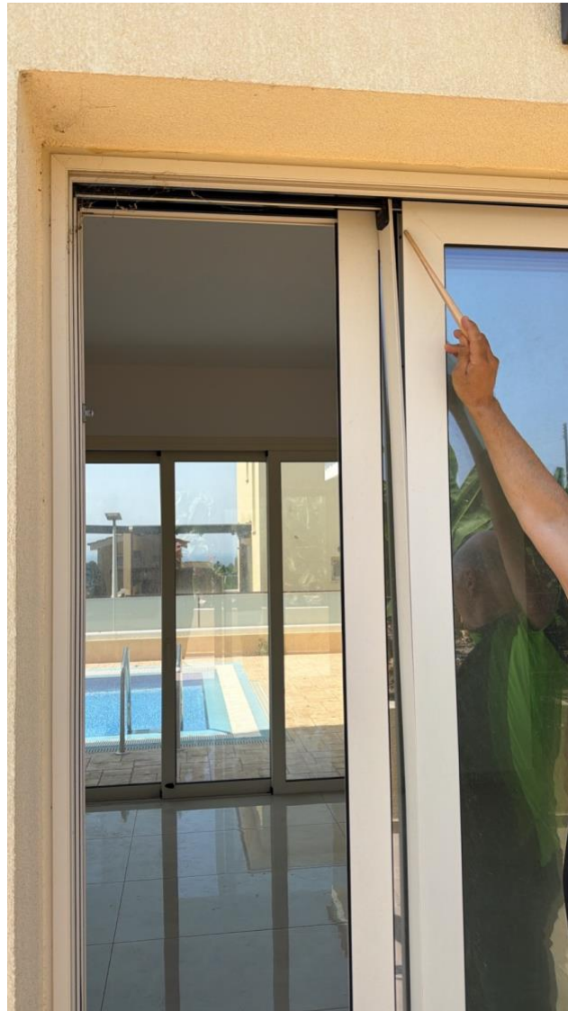
Figure 28. Open junction at the upper corner of the kitchen-to-backyard aluminium sliding-door frame.
