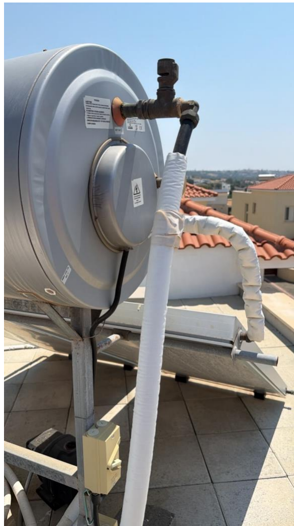
Figure 61. Roof-mounted solar hot-water equipment.
