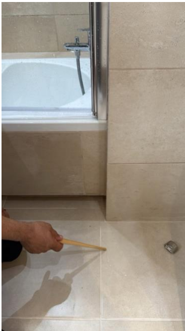
Figure 39. Water visible on the floor adjacent to the shared-bathroom bath/shower enclosure after testing.
