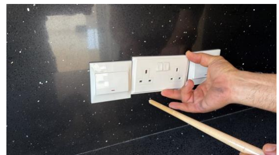
Figure 33. Further kitchen switch requiring secure fixing.
