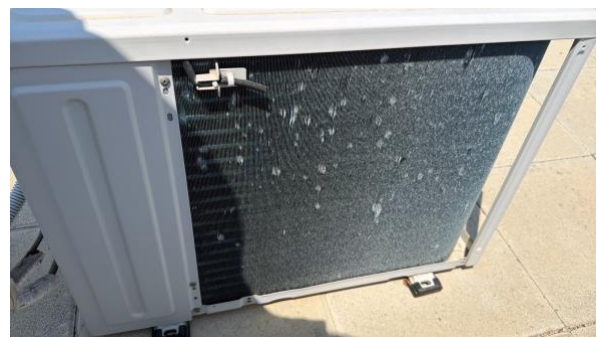
Figure 57. Further condenser coil fin damage.
