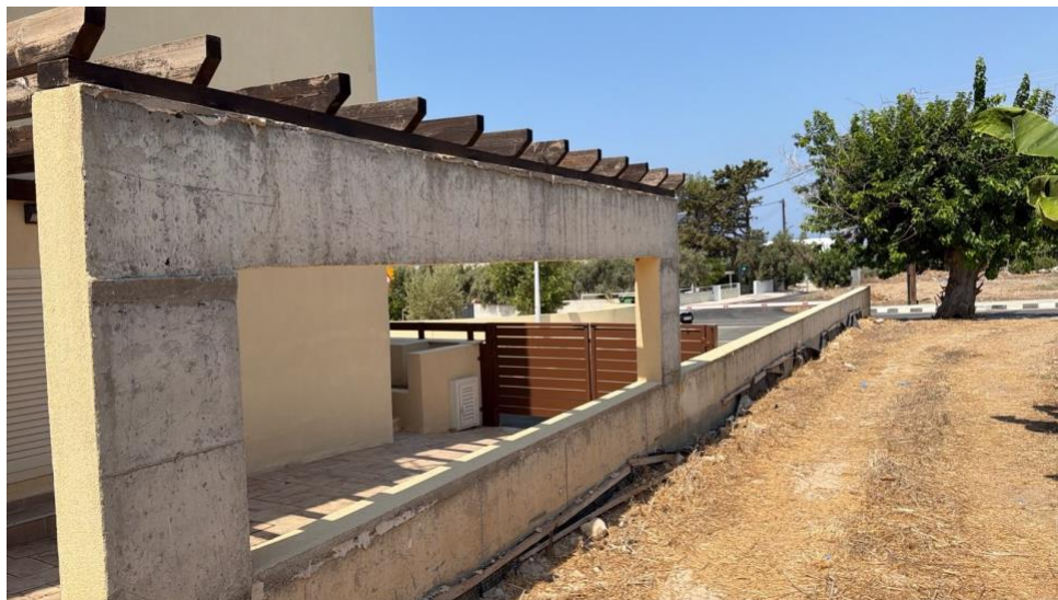
Figure 8. Unfinished exposed concrete face to the pergola support structure at the neighbouring side.
