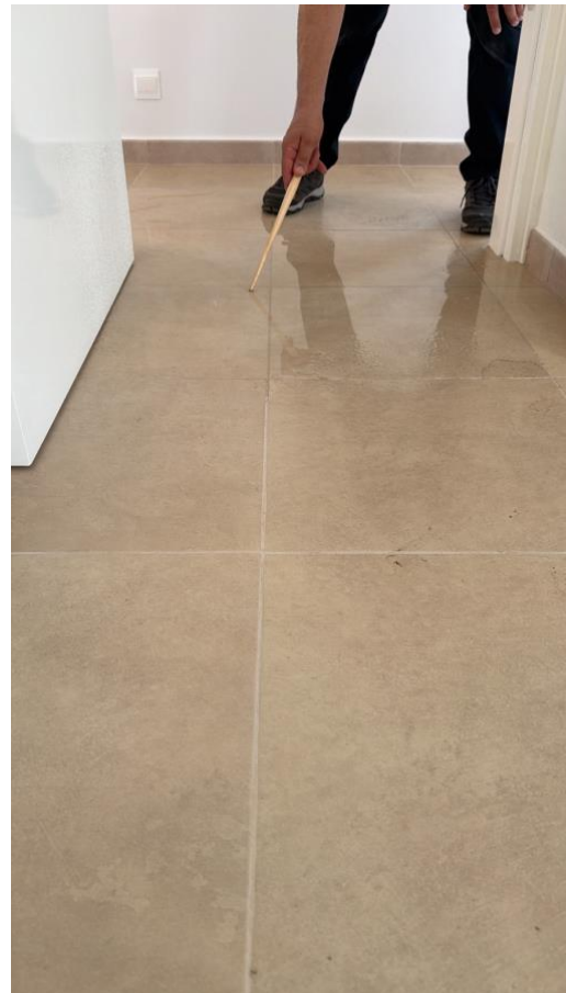
Figure 51. Condensate water discharged internally onto the middle-bedroom floor during testing.
