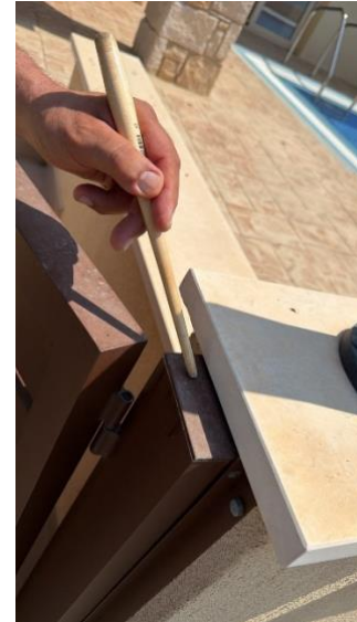
Figure 14. Missing cover to the gate finishing element.
