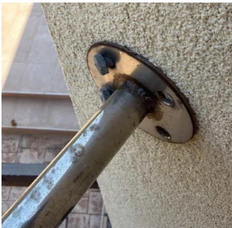
Figure 11. Further view of a roof-access ladder fixing showing incomplete anchorage.
