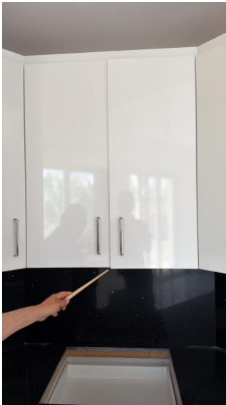
Figure 29. Misalignment between adjacent kitchen cabinet fronts.
