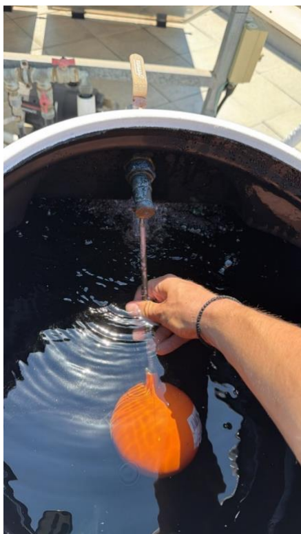
Figure 62. Water-storage tank internal float-valve check. condensers and water-storage tank.
