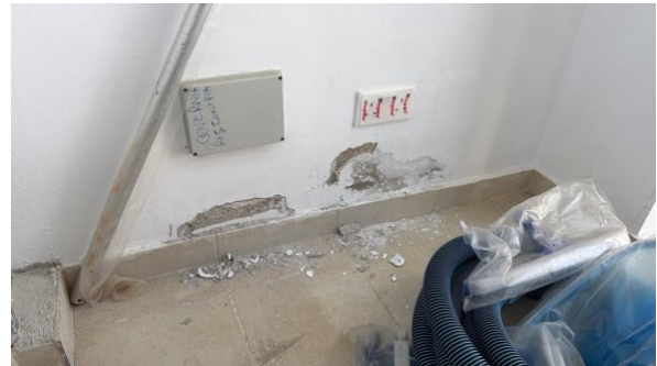
Figure 4. Internal finish deterioration on the corresponding wall.
