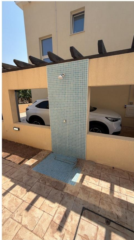
Figure 21. Outdoor pool shower tested during the inspection.
